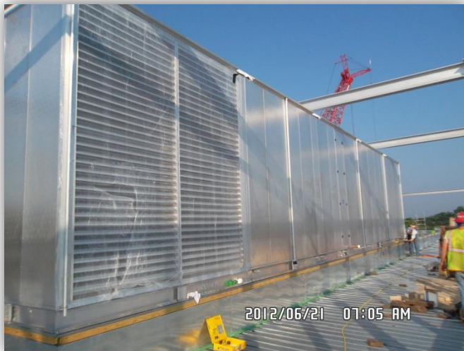
Roof top AHU with curbs - Taken by Derek Stoecklein
